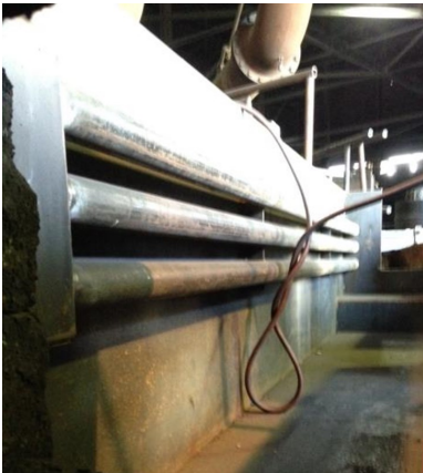
Internal Air Cooling
