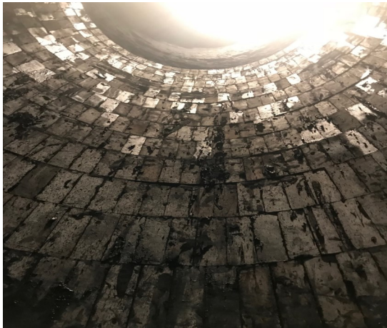
Arch Brick—DuraLast NB SiC - Lower Stack
